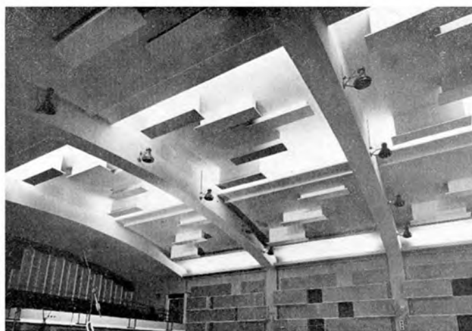
Acoustic treatment of Maida Vale Studio One (home of the BBC Symphony Orchestra). The scattering elements on the ceiling, and boxes on the walls, break up the sound waves
