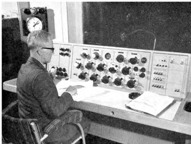
Studio 8 Broadcasting House: This is the desk that was used for the recording described in the text. Note that rotary faders are used; they can be switched to one or other of two group faders, if it is necessary to fade more than two at once. The studio manager is setting one of the echo-mixture switches, and above these are the "distort" switches. The microphone is for talkback to studio or recording room.
